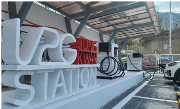
V2G charging station in Busan JungKwan Energy
